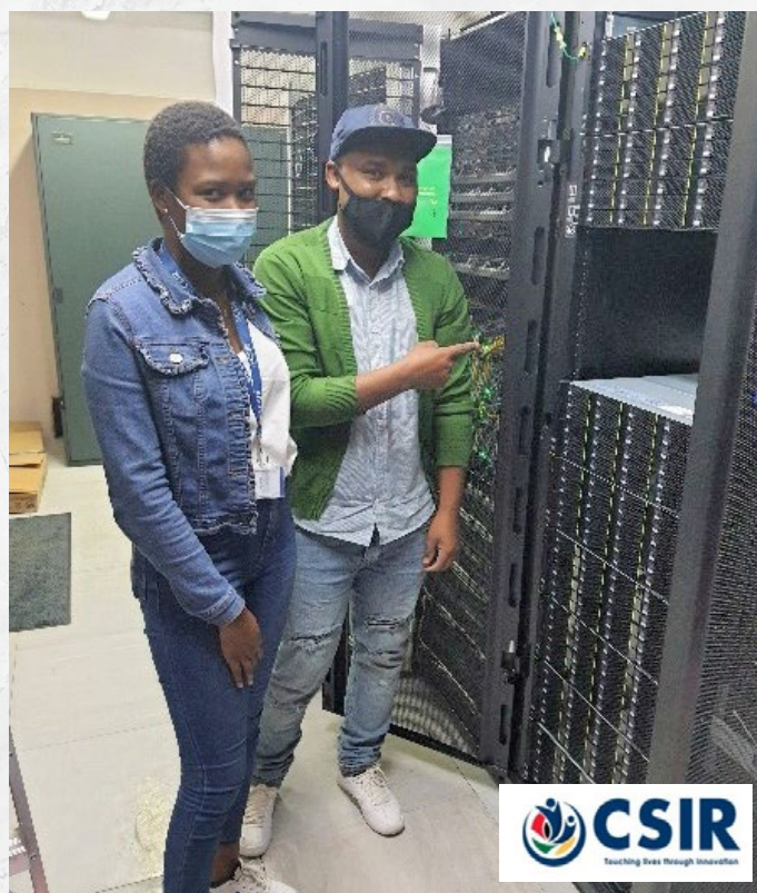
Figure 1: Interns racking and stacking servers, cabling and networking
