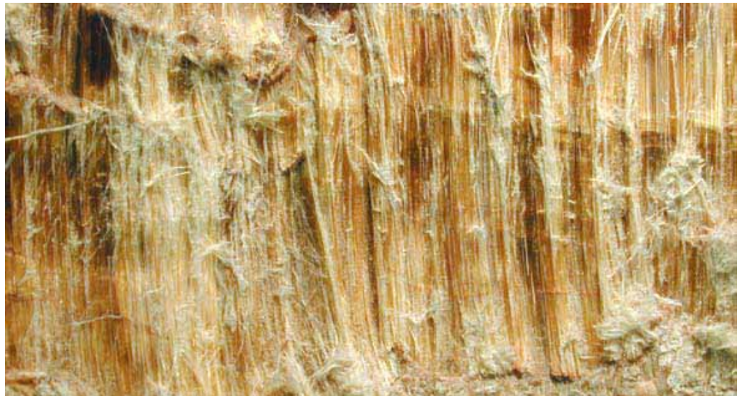
Asbestos deteriorates over time, leading to the possibility of inhalation of asbestos fibres which could lead to a range of pulmonary diseases such as asbestosis.
