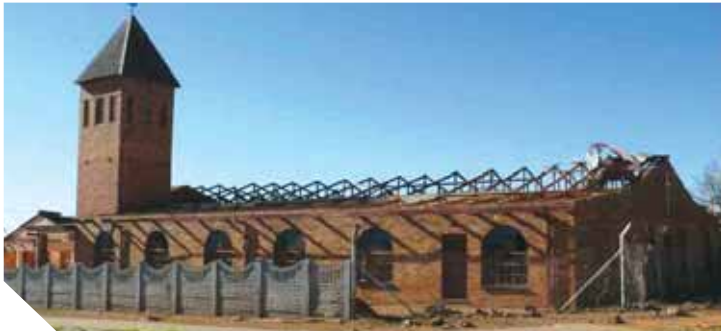
Figure 20: Roof blown off during Matlosana Wind Storm
