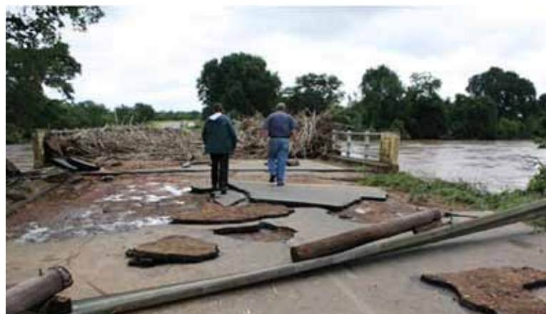
Damage to the Nwanedzi Bridge after flooding.
