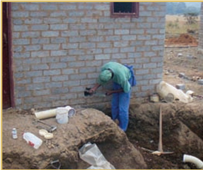
Gauteng: Mogale City Local Municipality, Magaliesburg: Blaauwbank Bulk Services to Housing Project
