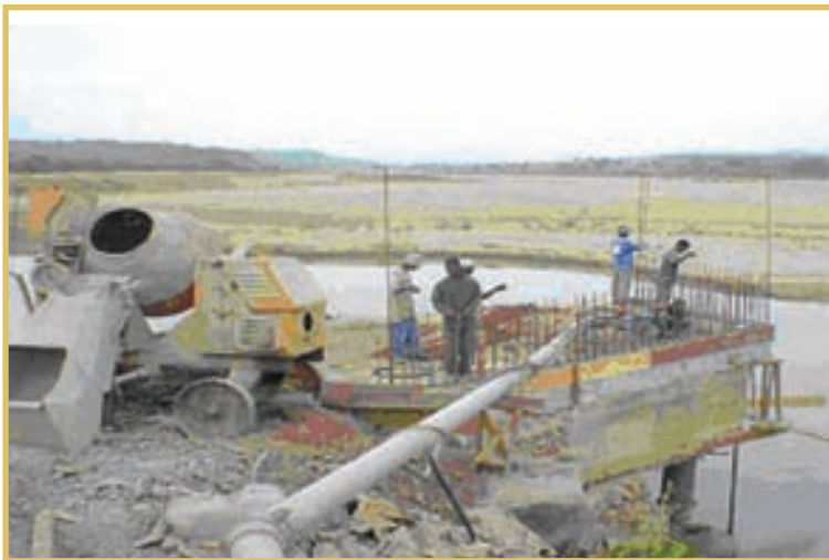
Eastern Cape: Ndlambe Municipality (Port Alfred): Mimosa/Nemanto - Upgrading of the Water Purification Works
