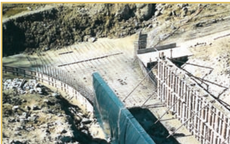
Northern Cape: Upington Water Purification System
