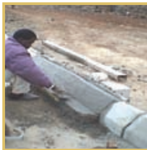
Gauteng: Ekurhuleni Municipality, Winnie Mandela Park: Construction of access streets and stormwater drainage
