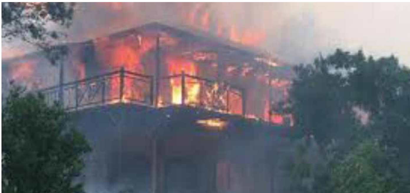
FIGURE 15: One of the properties damaged during the June 2017 Knysna and Plettenberg Bay fires, Western Cape fires.
